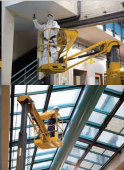
INDOOR FINISHINGS (electrical, lighting, plumbing, painting, HVAC, piping, fire detection systems, etc.)
